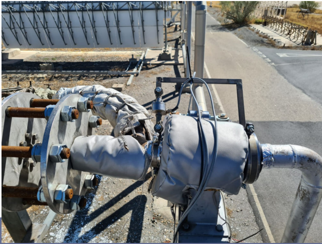
Mounted load cells on URSSA-trough at PSA
