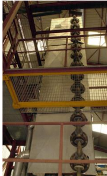
Figure 6. Solar Multi-Effect Distillation installation (SOL-14)
